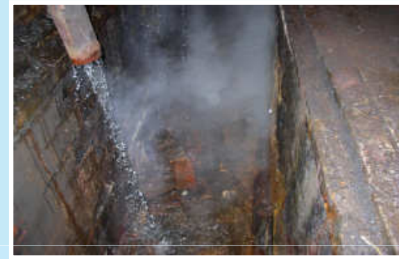
Gutter in need of rehabilitation
