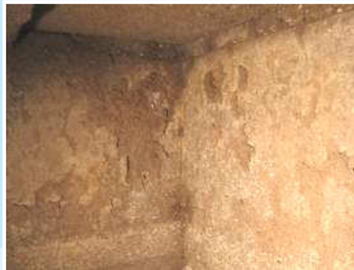
Container in need of rehabilitation
