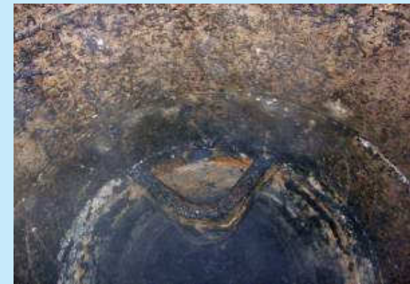
Seperator in need of rehabilitation
