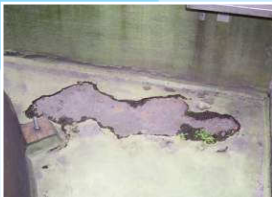
Floor in need of rehabilitation
