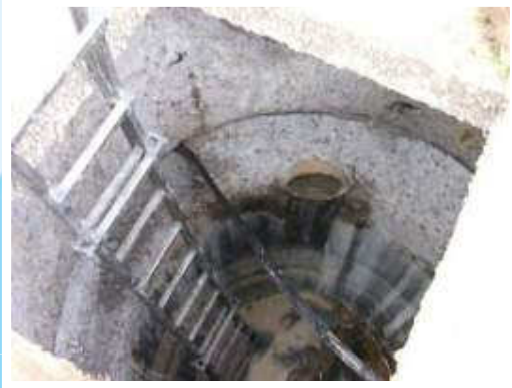
Manhole in need of rehabilitation
